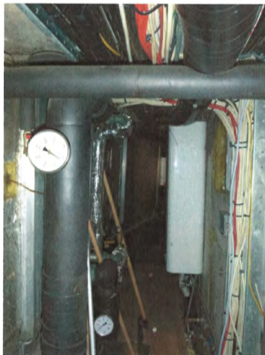
Blick in Klimazentrale am Ponton
